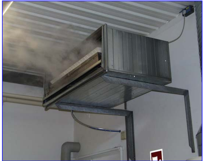
Picture of aerosols during direct room humidification with direct room humidifier DRF42. Humidification capacity 25 kg/h.
