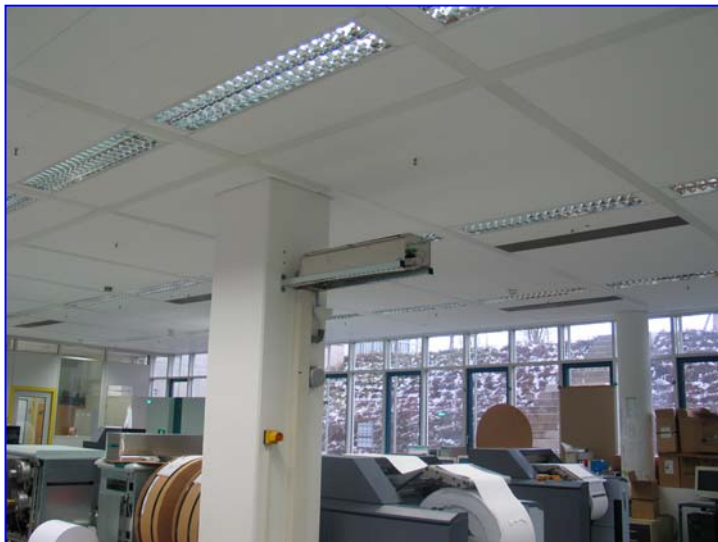
RB/P-D build in for direct- room-humidification inside a print office. Location: South Germany
