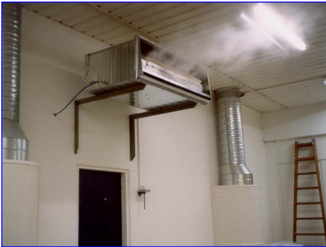
Direct room humidification in a printing house in Copenhagen.
