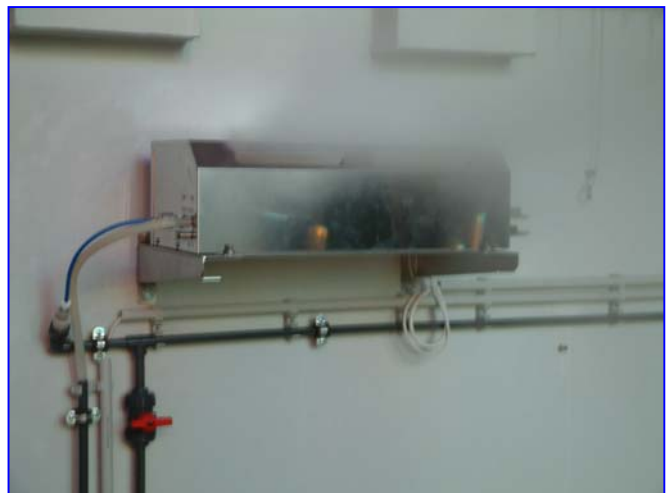
Direct humidification embedded in a church.
